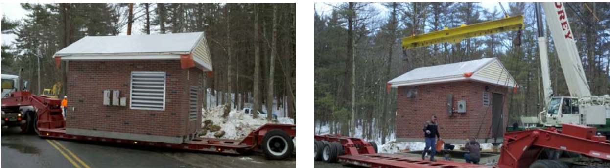
(Brookline St. pump station control building being delivered and set on cast-in-place wet well)
