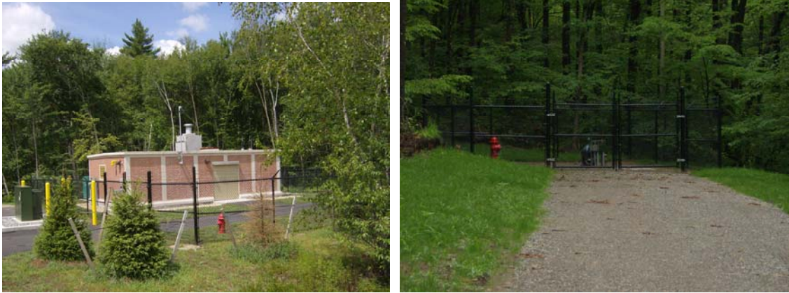
(left: finished Nashua Road Well pumping facility; right: completed Nashua Road Well)
