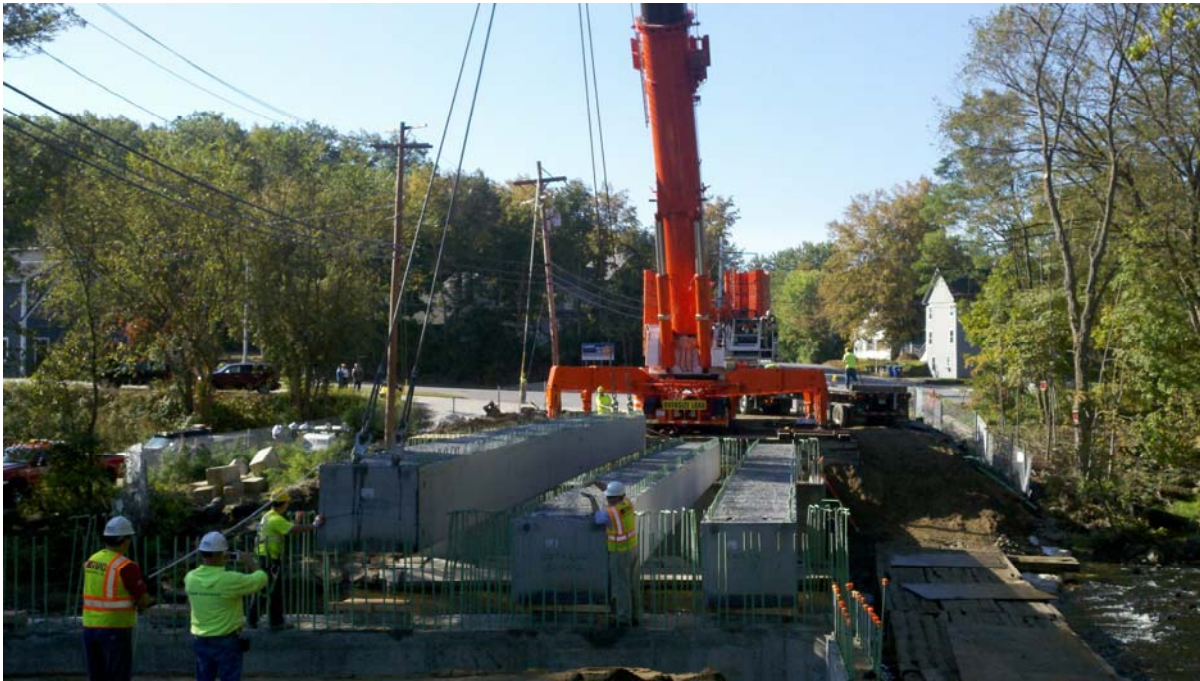
(Precast concrete box beam sections being installed with a 600 ton crane at the Mill Street Bridge project)
