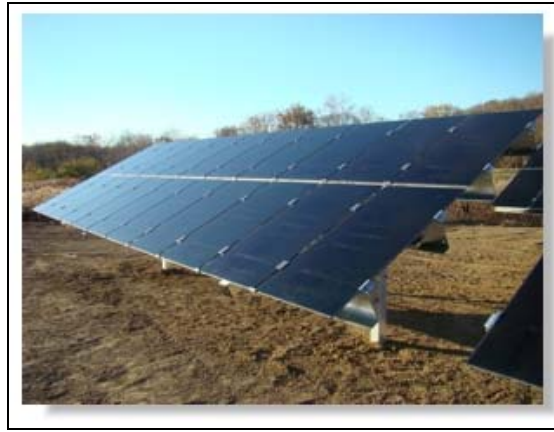
Typical ballasted, rack mounted solar PV panel.
