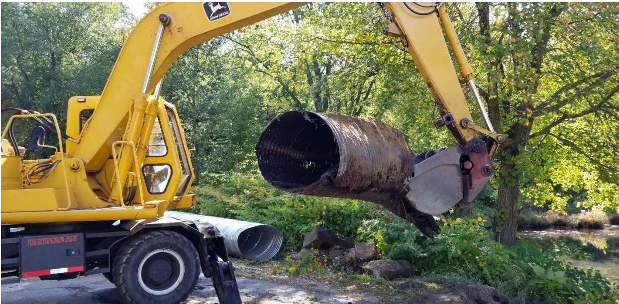
Highway Department removing a section of the old culvert pipe as part of the Leighton St construction project.
