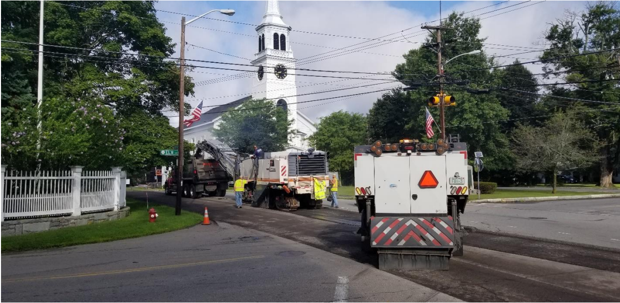
Brox Industries milling out the pavement at the Main/Elm/Park intersection as part of the Townsend St construction project.
