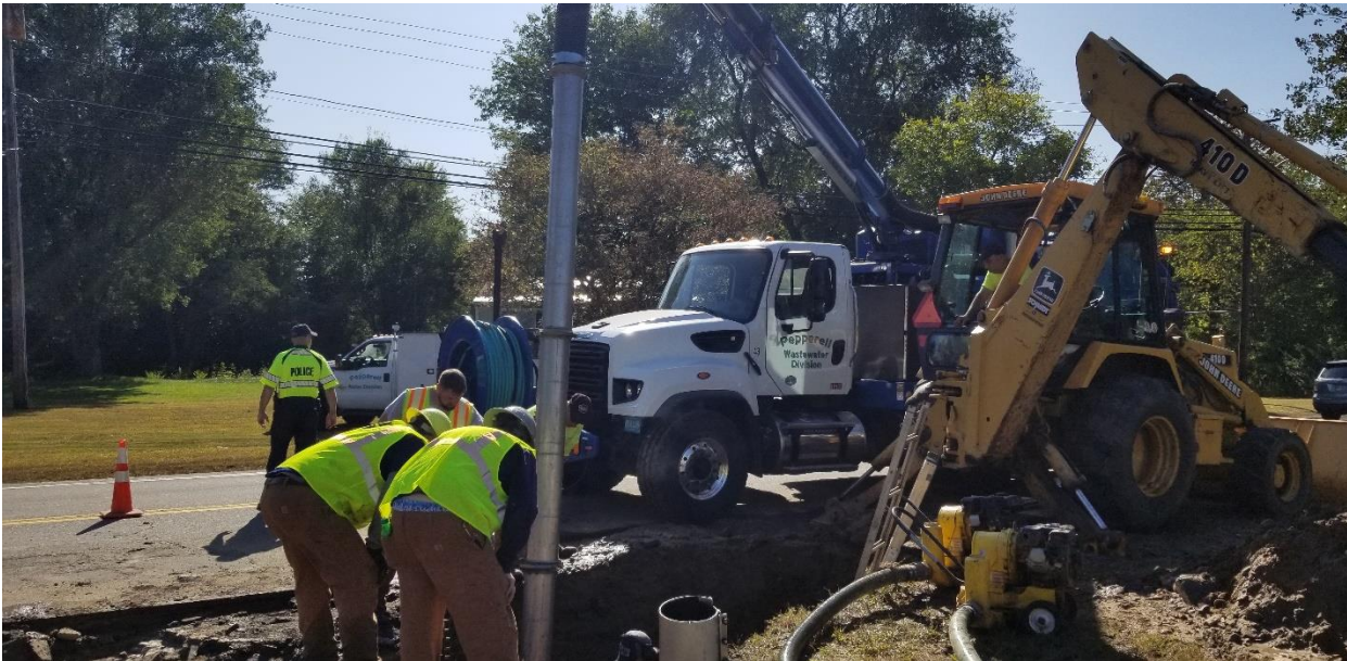
Water, Sewer and Highway crews and equipment working together to repair water main break on Lowell Road.
